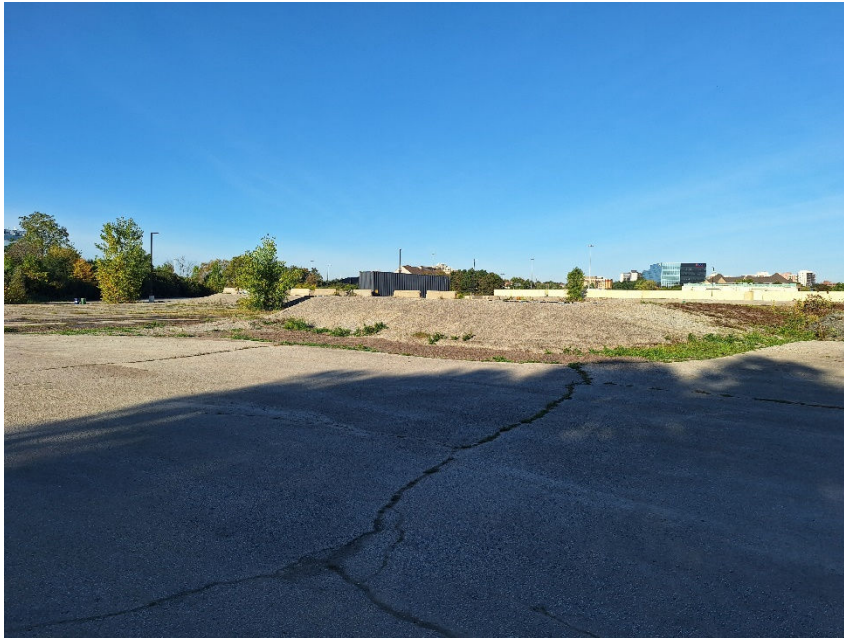
Image 15: View of the variable elevations of the concrete and asphalt surfaces in the central part of the subject property.
