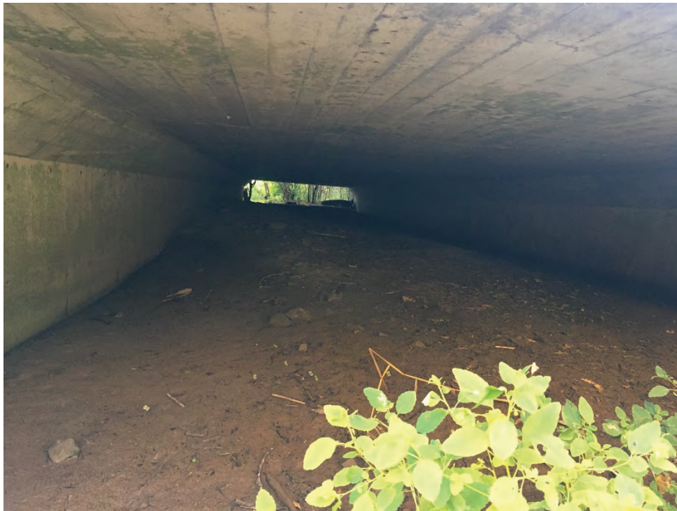
Photo 4 - Sediment Deposition Through the Private Road 2 Culvert
