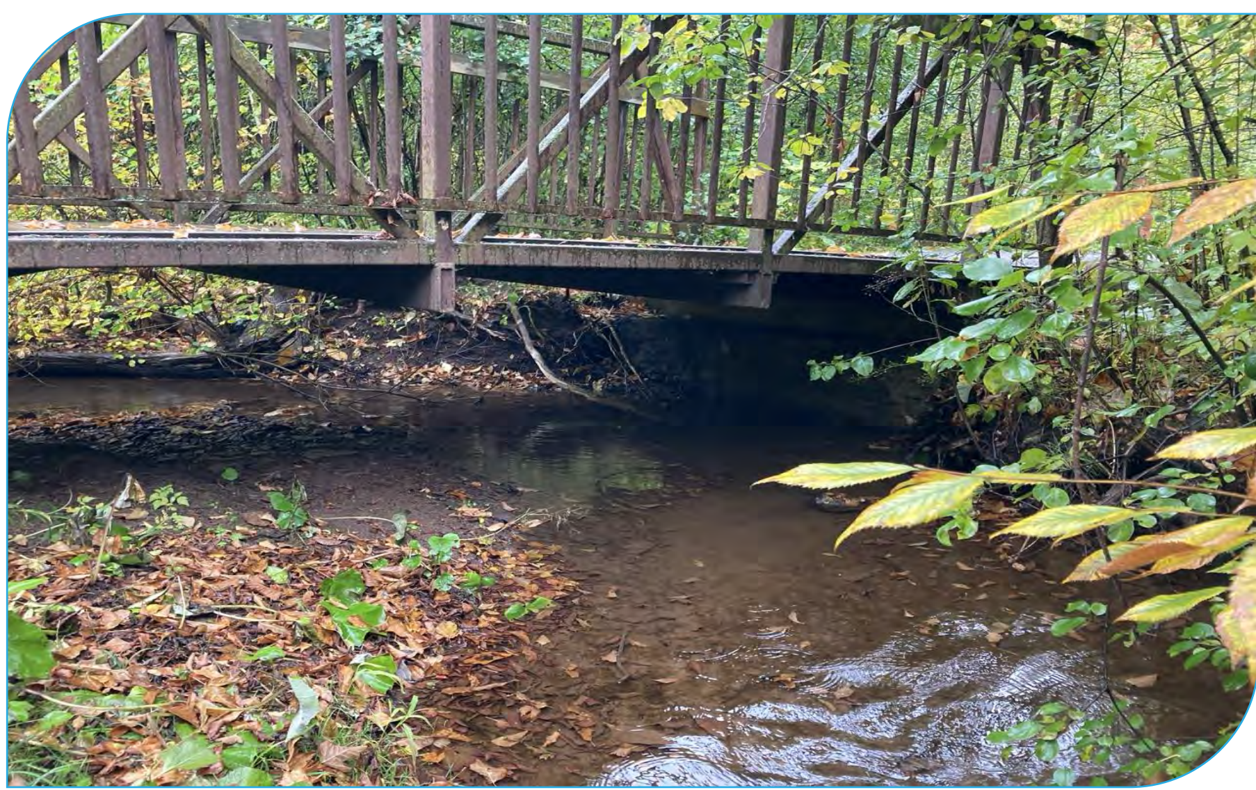
Site: E21 Score: 43 Issue: Erosion around pedestrian bridge; footing exposed within the channel. No damage to the concrete footing currently. Risk: Trail infrastructure including pedestrian trail and pedestrian bridge crossing Length: < 10 m
