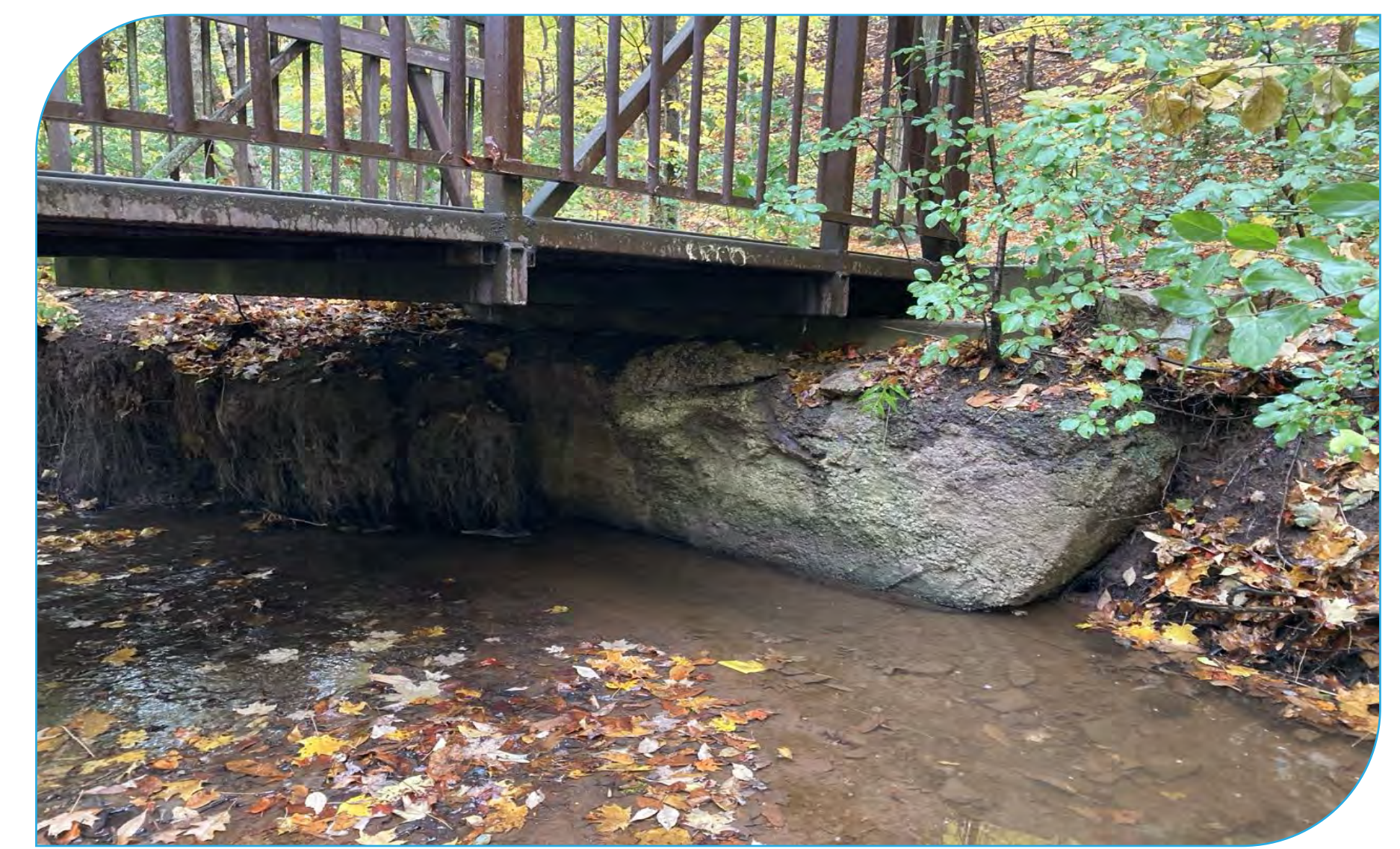
Site: E20 Score: 43 Issue: Erosion around pedestrian bridge crossing; footing exposed on the outer meander bend. Risk: Trail infrastructure including pedestrian trail and pedestrian bridge crossing Length: < 10 m
