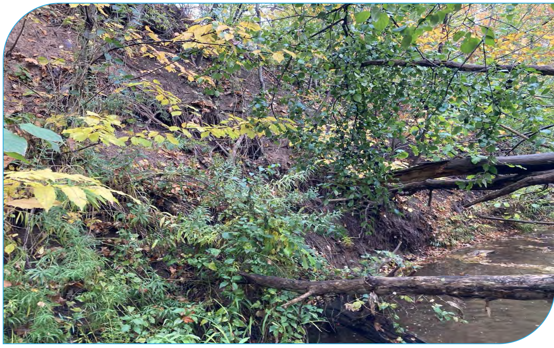
Site: E23 Score: 37 Issue: Valley wall contact; eroding valley slope Risk: Potential risk to pedestrian trail system and private property Length: 10 – 20 m
