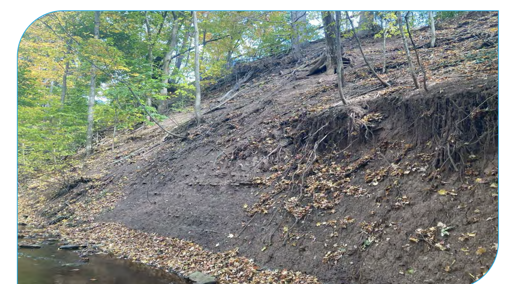
Site: E4 Score: 65 Issue: Valley wall contact and slope erosion. Gabion protection near upstream end of erosion is in poor condition (bottom tier corroded/emptied) Risk: Private property Length: > 100 m
