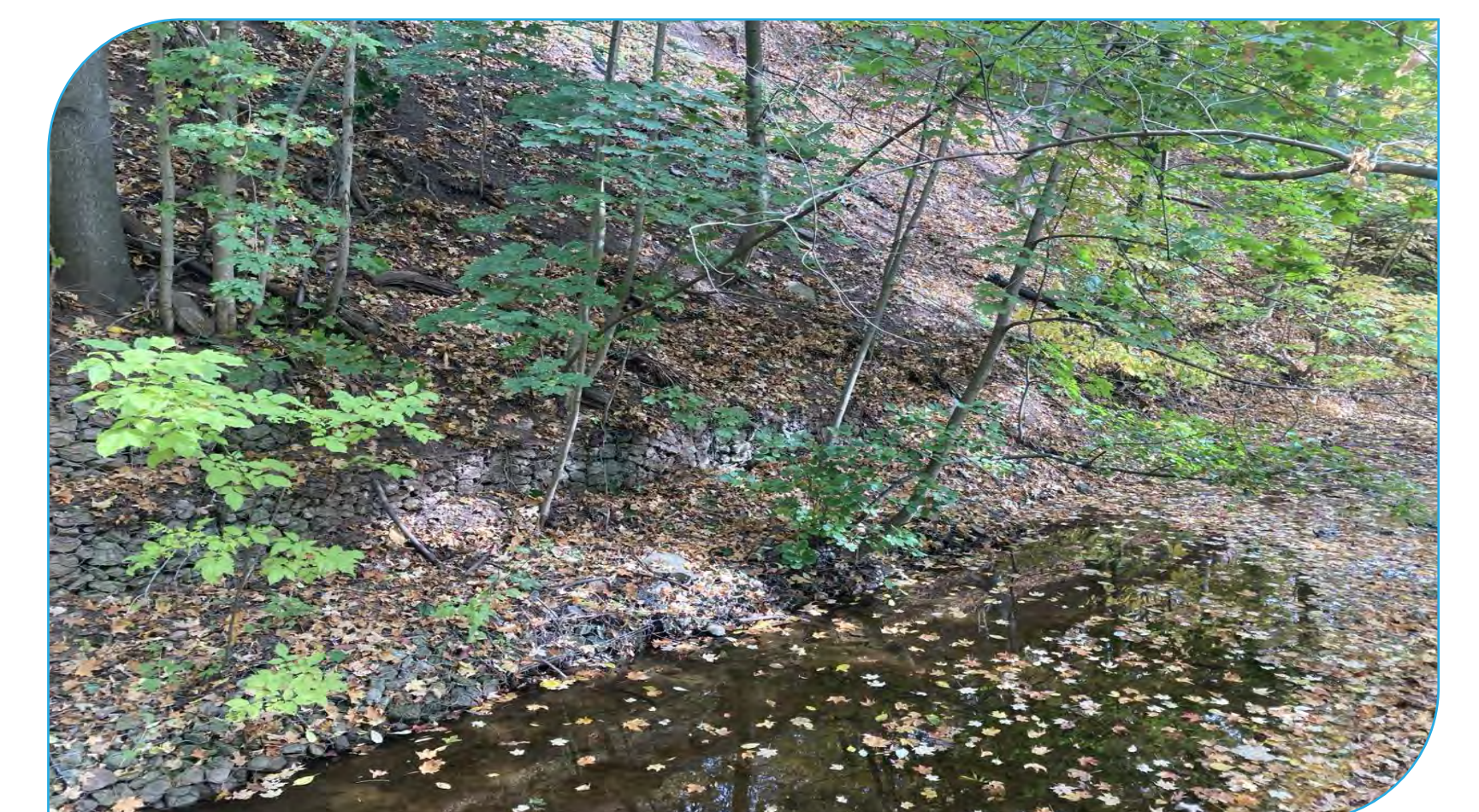
Site: E24 (new site) Score: 59 Issue: Valley contact/slope erosion. Gabion toe protection - fair condition (functioning, some wire failure at toe) Risk: Private property Length: 20 – 50 m
