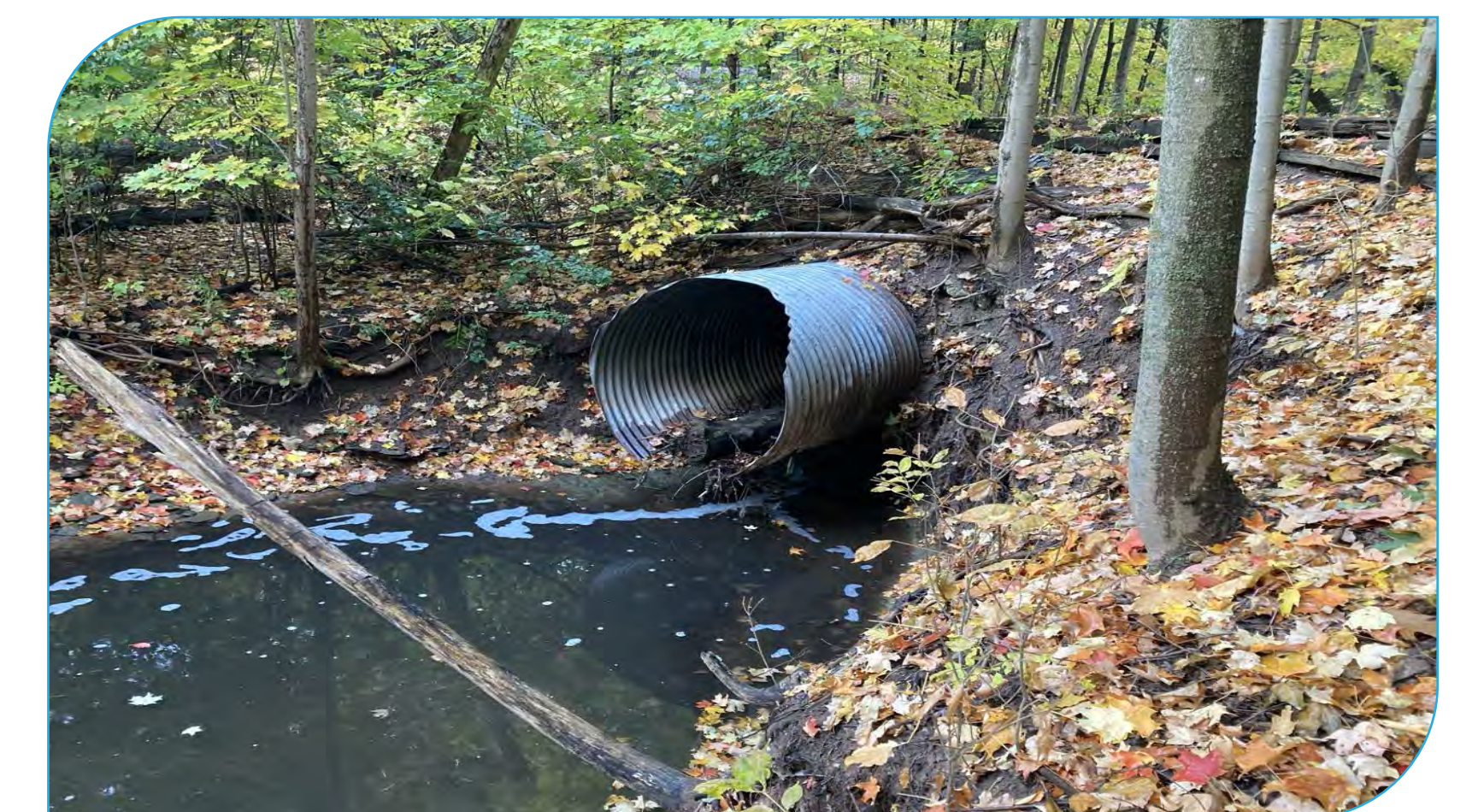
Site: E11 Score: 79 Issue: CSP culvert below trail, bottom corroded. Scour pool downstream. Buried sanitary sewer. Risk: Critical infrastructure (sanitary sewer), pedestrian path/crossing Length: 20 – 50 m
