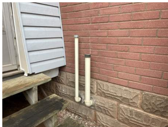
Photo 12: View of the vent and fill pipe for the AST located on the exterior north facing wall on the southwest portion of the Site building.
