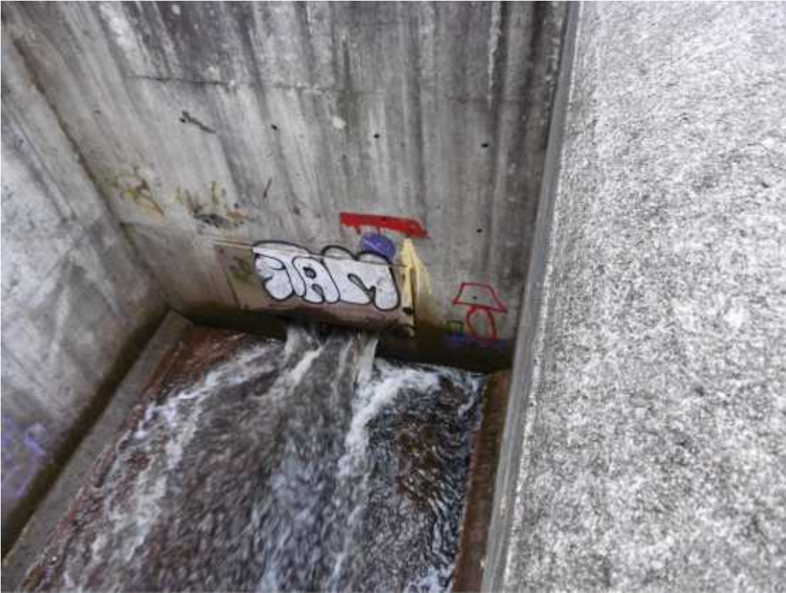
3. Inside View of Orifice Plate (Covering approx. 2/3 of first stage control)
