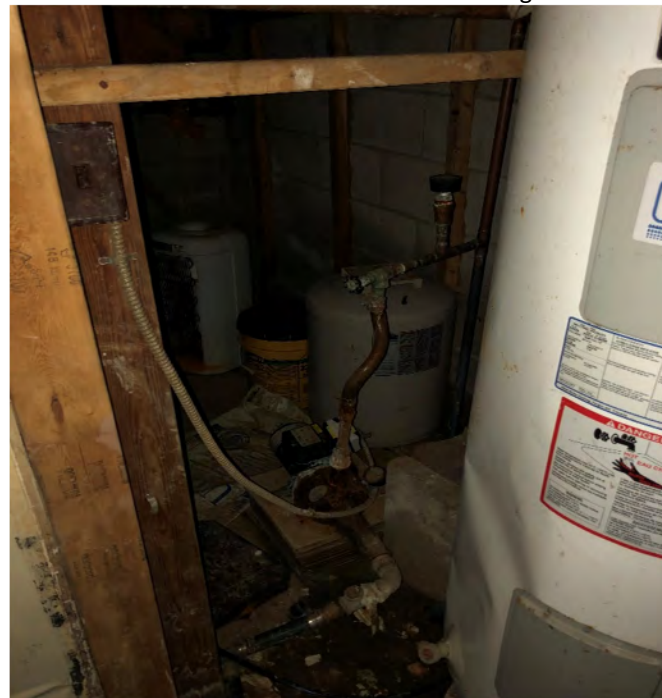
Photo 8: Sump Pump in the interior of the Site Building
