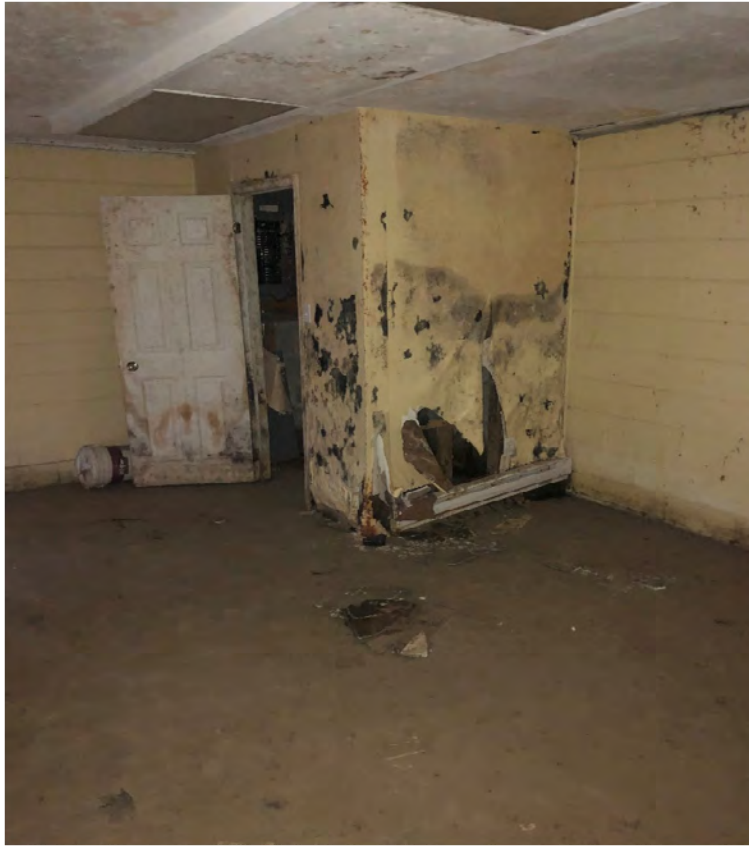
Photo 9: Interior Water Damage of Site Building
