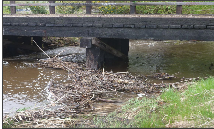
Debris in Creeks
