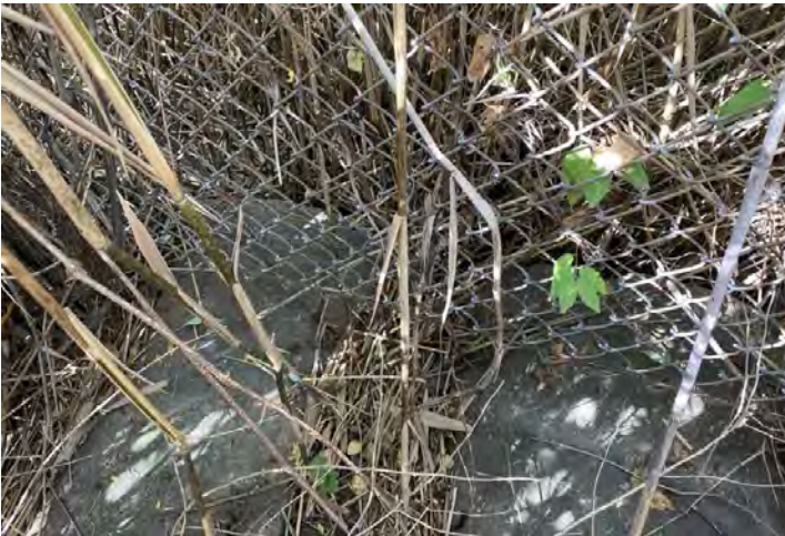
Photo 3: Conditions of the unregulated drain twin culvert segment at property fence line near SSRE. Photo facing NW/Down.
