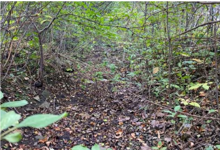
Photo 5: Conditions of the unregulated drain south of the Davis Rd. culvert crossing Photo facing NW (upstream).
