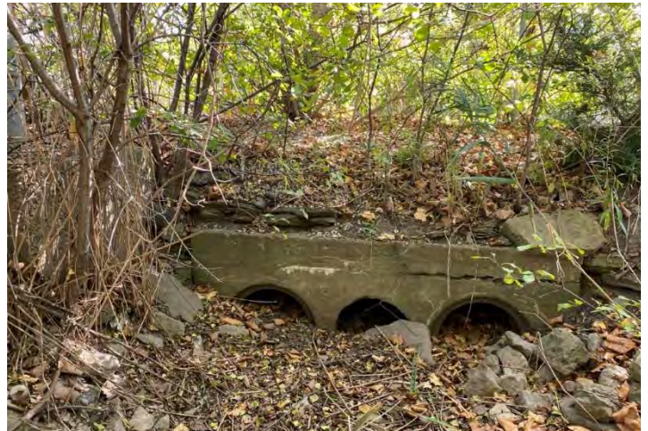
Photo 4: Conditions of the unregulated drain at the Davis Rd. culvert crossing. Photo facing SE (downstream).
