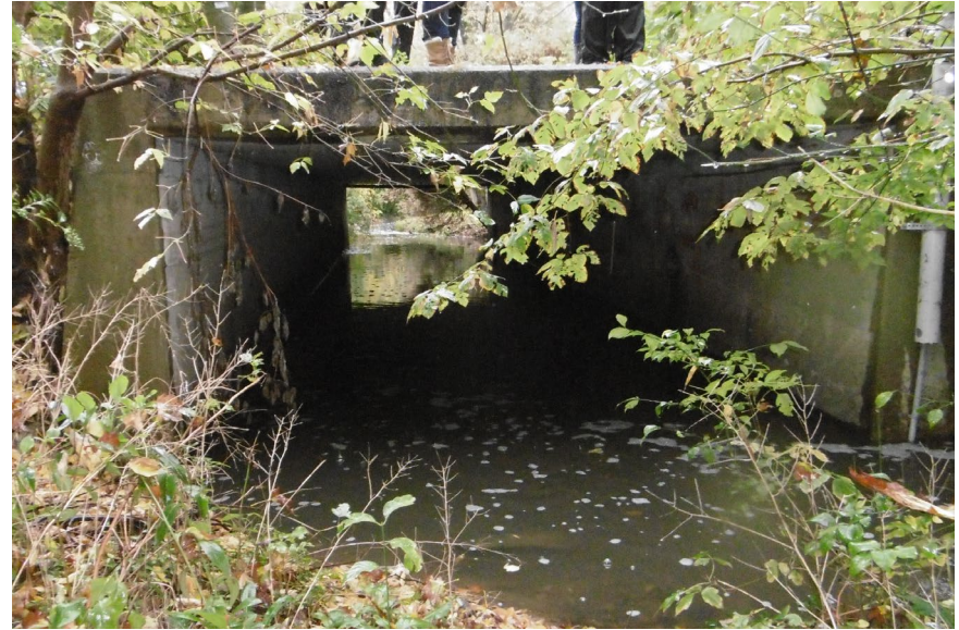
2: U/S Face of Morrison Road 3.7m x 2.05m Conc. Box Culvert, Station 878.3941
