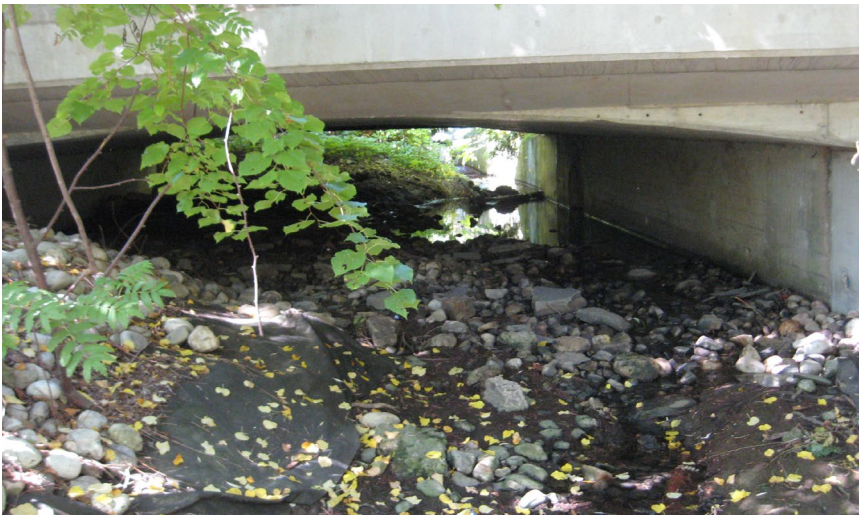
3: D/S Face of Linbrook Road 7.3m x 1.1m Conc Arch Culvert, Station 120.4545
