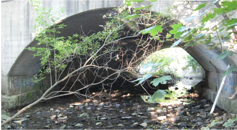
1: D/S Face of Lakeshore Road 7.9m x 3.2m Conc. Arch Culvert, Station 354.4469
