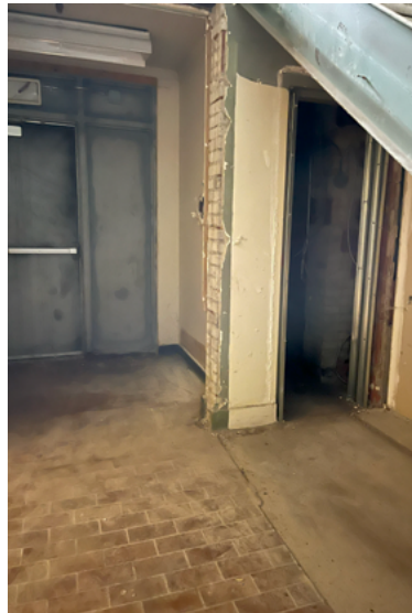
Metal door at the main entrance is in poor condition; missing drywall showing brick underneath (ERA, 2024).
