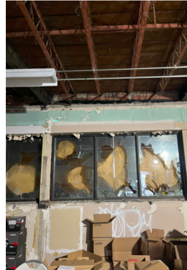
Windows in defective condition showing broken glazing (ERA, 2024).
