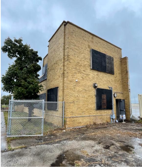
Looking east toward the western elevation of the office building (ERA, September 23, 2024).
