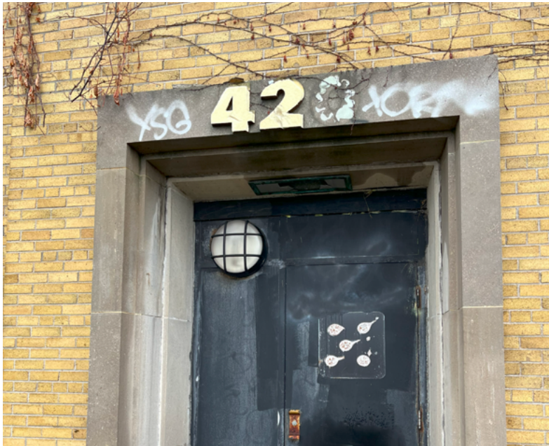
Stone portico main entrance is in fair condition with areas of poor condition showing delamination, mortar loss, staining, and graffiti (ERA, 2024).
