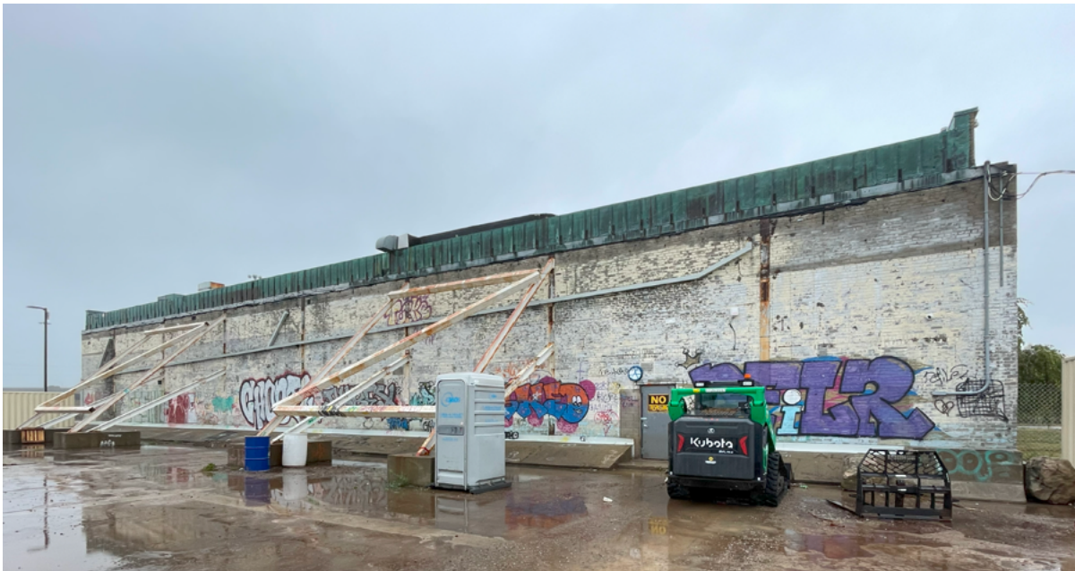
Looking north toward the southern elevation of the office building. Following the demolition of the factory buildings in 2011, steel shoring was installed to support what was originally an interior wall (ERA, September 23, 2024).
