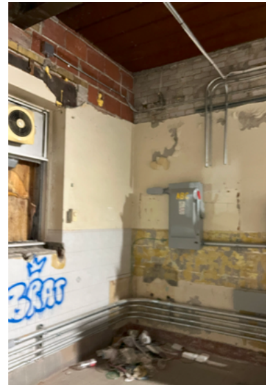
Missing drywall showing brick and terra cotta tile underneath (ERA, 2024).
