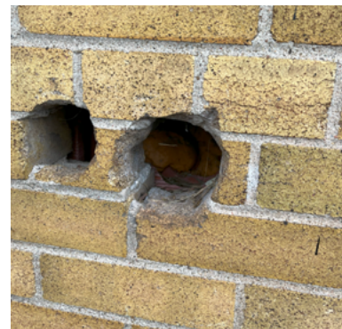
A section at the base of the brick wall on the south elevation showing signs of destructive testing (ERA, 2024).
