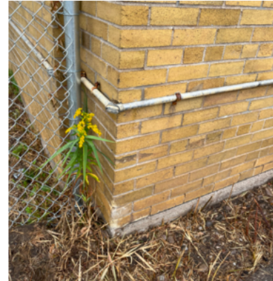
Bricks in fair condition with localized areas of poor condition (ERA, 2024).
