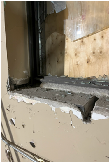
Missing drywall showing concrete block underneath; windows in defective condition showing broken glazing (ERA, 2024).
