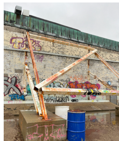
Bricks on south elevation and temporary steel shoring is in poor condition (ERA, 2024).
