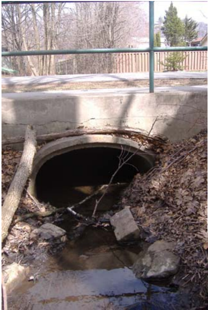
Photo 38: Upstream face of culvert at Woodhaven Park Drive. Note partial obstruction.
