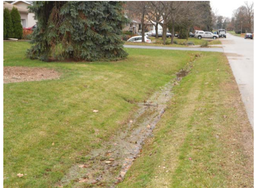
Photo 16: Looking upstream along west ditch of Westminster Drive. Note standing water in ditch.
