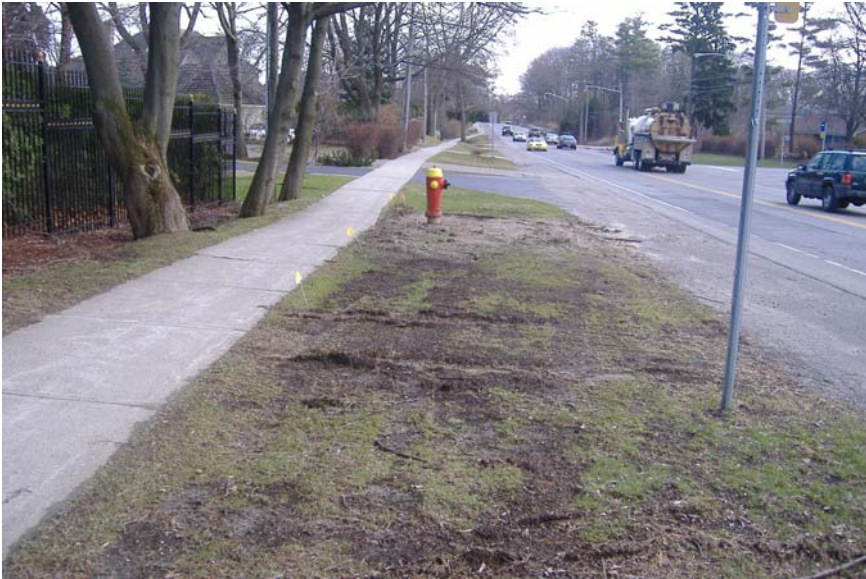
Photo 87: Looking west along south side of Lakeshore Road. Note lack of ditch and erosion on side of road.
