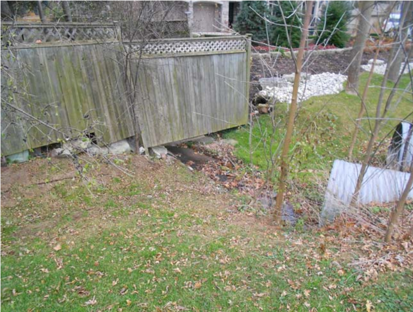
Photo 21: Looking at downstream face of culvert crossing of Old Lakeshore Road. Note flow obstruction (wooden fence).
