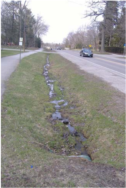
Photo 80: Looking east along north ditch of Lakeshore Road. Note standing water and erosion/rutting.
