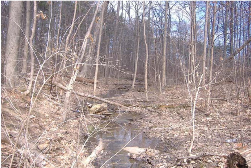
Photo 55: Looking downstream at open channel behind Hixon Street. Note bank erosion and tree debris.
