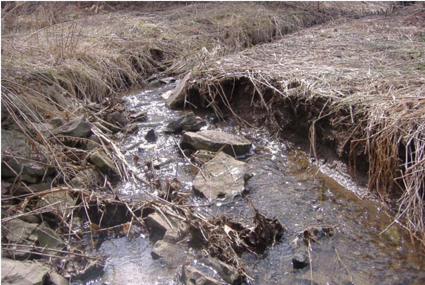
Photo 75: Looking upstream from Lakeshore Road culvert. Note bank erosion.
