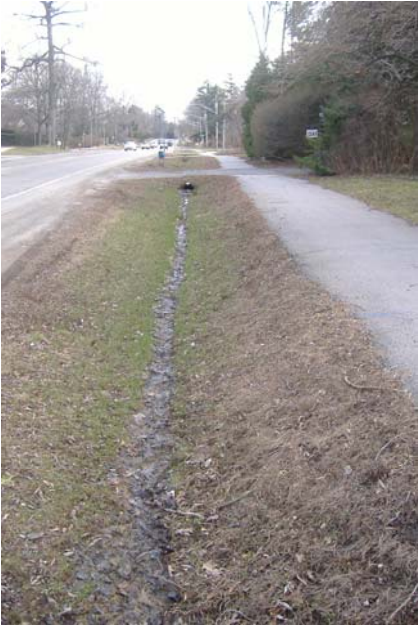
Photo 84: Looking west along north ditch of Lakeshore Road. Note standing water and erosion/rutting.
