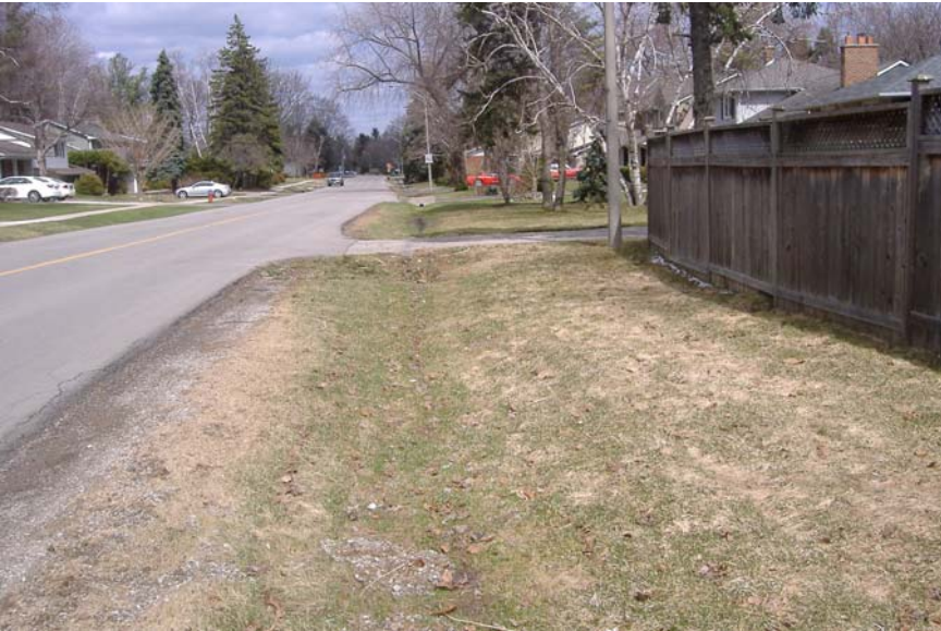
Photo 26: Looking east on south side of Hixon at Tracina. Note filled ditch/culvert.
