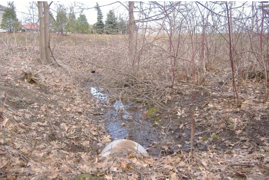
Photo 72: Looking downstream along channel behind Woodhaven Park Drive. Note minor bank erosion.
