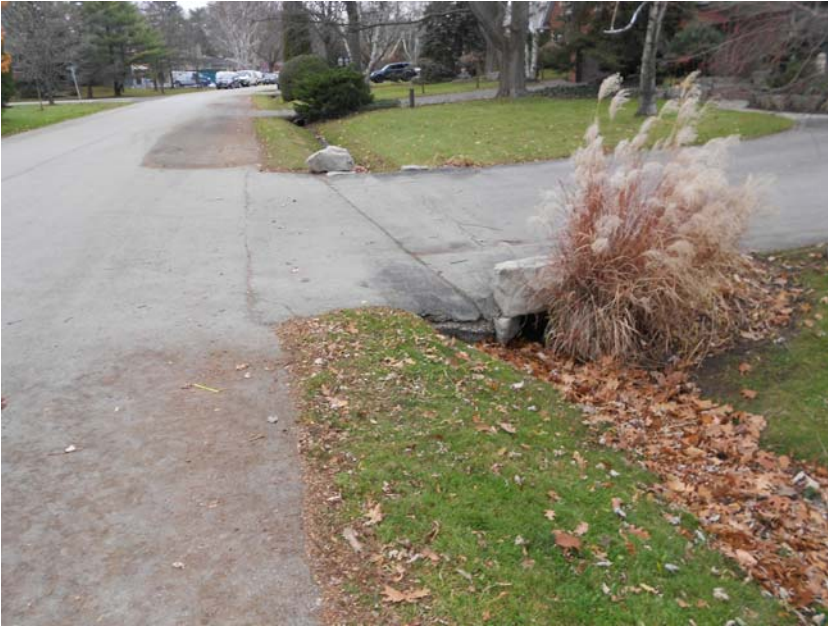
Photo 13: Looking upstream along east ditch of Westminster Drive. Note ditch plantings and culvert obstruction.
