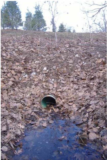
Photo 70: Undersized PVC culvert outlet on WWTP site. Note partial obstruction.
