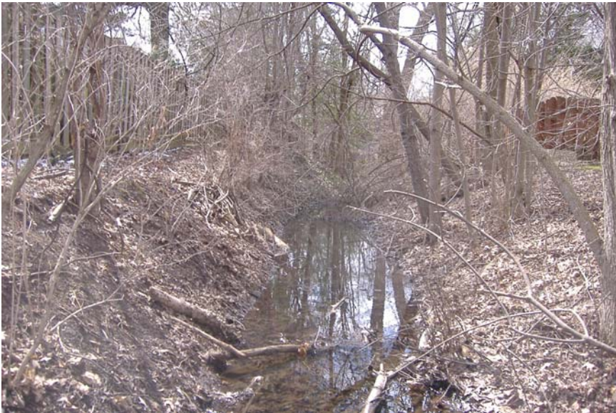
Photo 37: Looking upstream from Woodhaven Park Drive. Note minor bank erosion.
