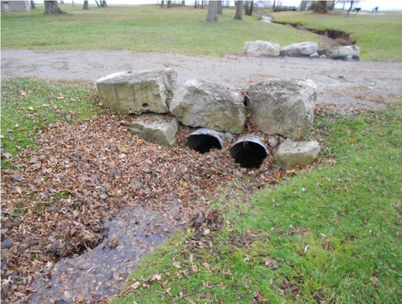
Photo 9: Looking downstream at culvert crossing. Note debris accumulation/blockage and standing water.
