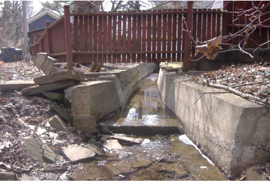
Photo 52: Looking upstream at concrete lined channel/storm outfall behind Hixon Street. Note debris accumulation.
