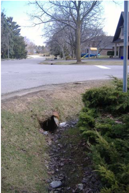
Photo 56: Looking downstream at partially crushed culvert at Selgrove Crescent and Woodhaven Park Drive.
