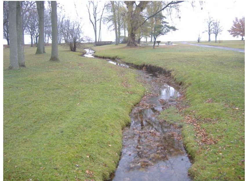
Photo 8: Looking downstream at channel from pedestrian culvert crossing. Note bank erosion and standing water.
