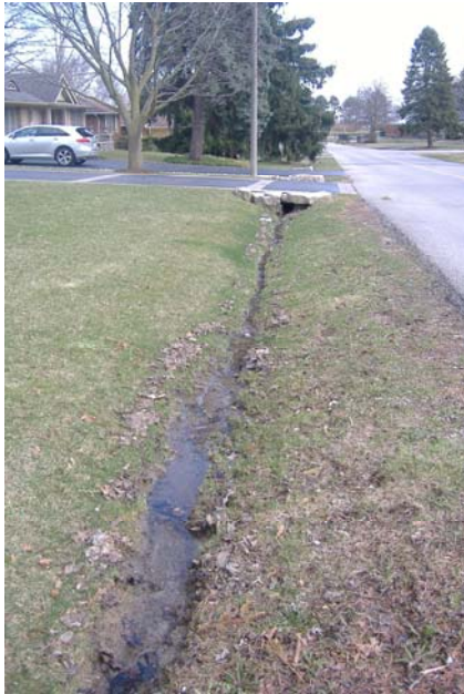
Photo 57: Looking south along east ditch of Woodhaven Park Drive. Note standing water and channel erosion/rutting.
