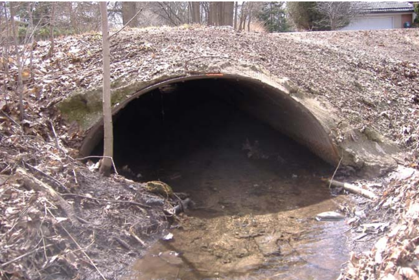
Photo 36: Downstream face of culvert at Woodhaven Park Drive. Note partial obstruction.
