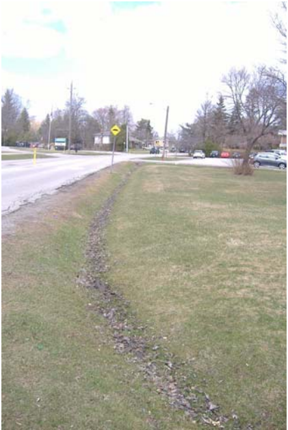
Photo 43: Looking east along Sedgewick Crescent. Note ditch erosion.
