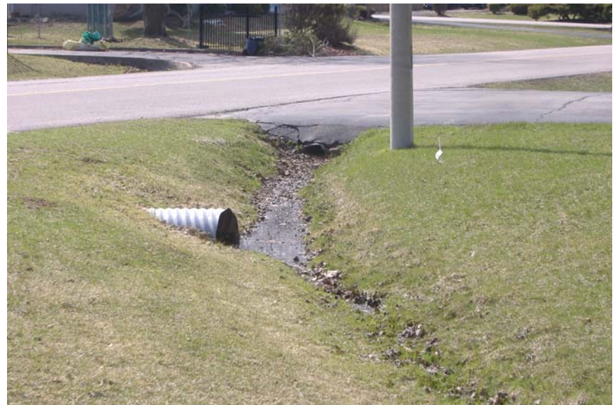
Photo 65: Looking north along east ditch of Woodhaven Park Drive at Lakeshore. Note standing water and partially crushed driveway culvert.
