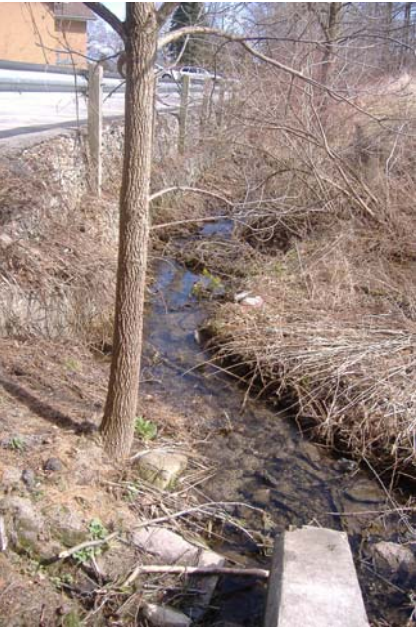
Photo 79: Looking downstream at open channel from storm sewer outfall at Lakeshore Road. Note bank erosion.
