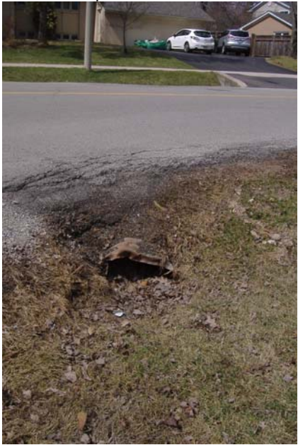
Photo 40: Downstream face of Sedgewick Crescent culvert. Note obstruction and crushing.
