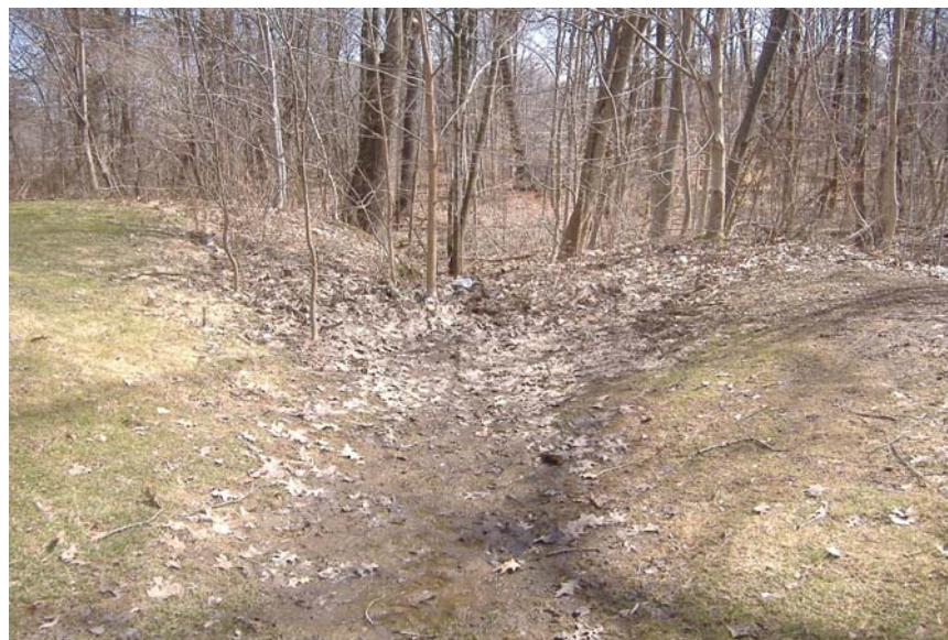
Photo 47: Looking downstream at ditch outfall to forest area. Note sedimentation.
