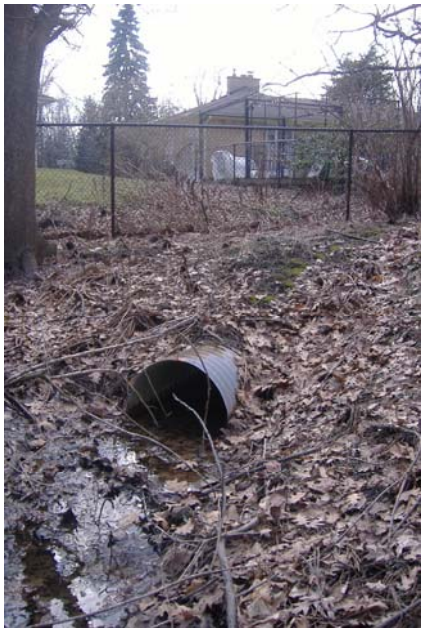
Photo 71: Storm sewer outfall behind Woodhaven Park Drive. Note partial obstruction.
