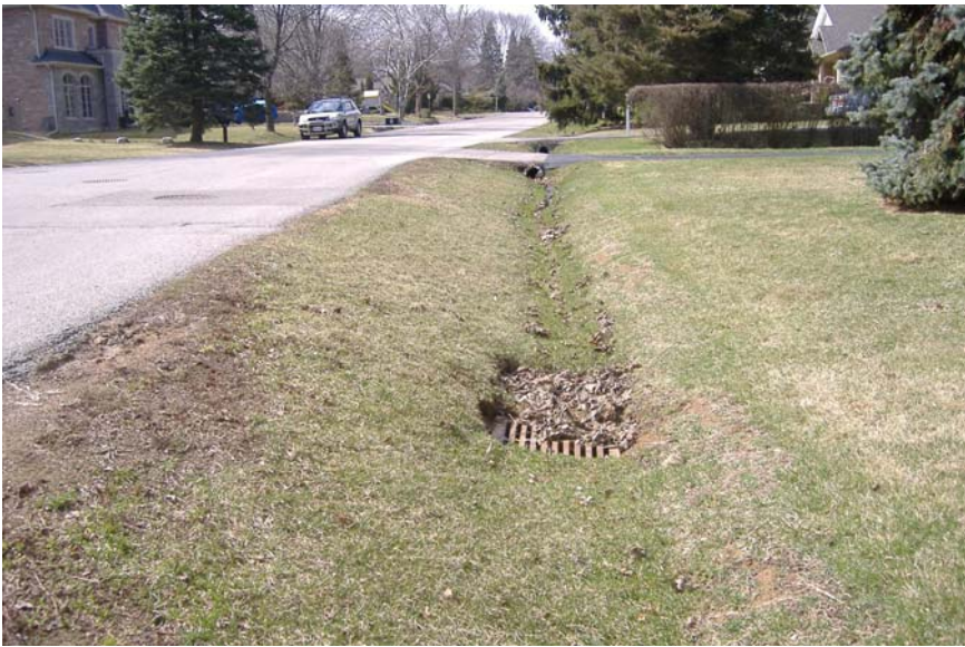
Photo 61: Looking north along east ditch of Woodhaven Park Drive. Note erosion around catchbasin.
