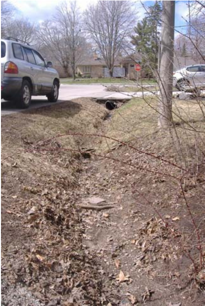
Photo 35: Looking upstream along Woodhaven Park Drive. Note channel erosion.
