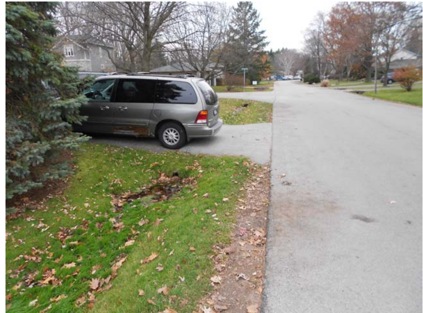
Photo 12: Looking upstream along west ditch of Westminster Drive. Note localized pooling and blocked culvert.
