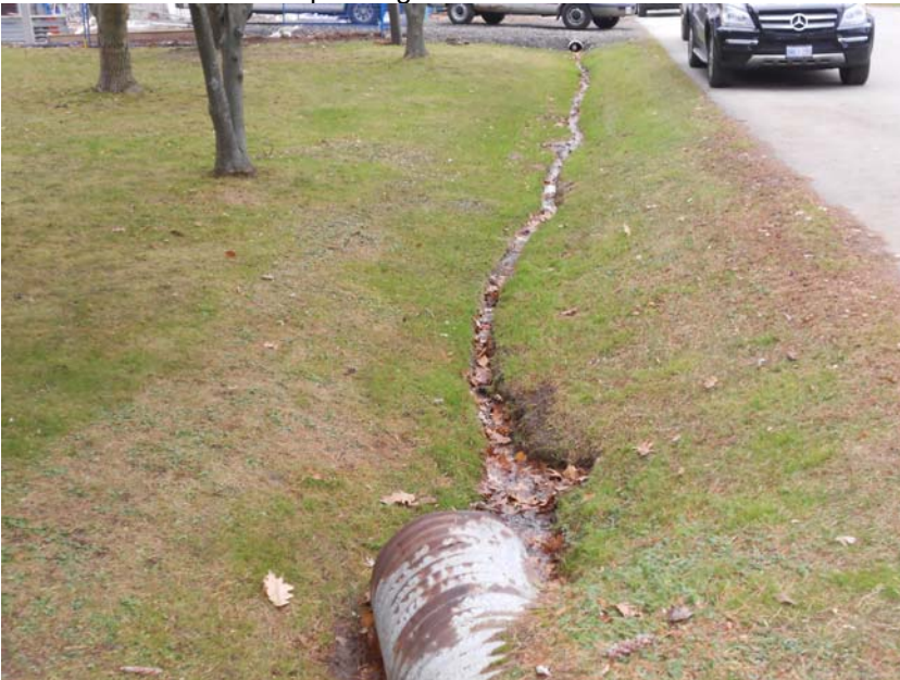
Photo 15: Looking upstream along west ditch of Westminster Drive. Note rutting erosion and skew culvert.
