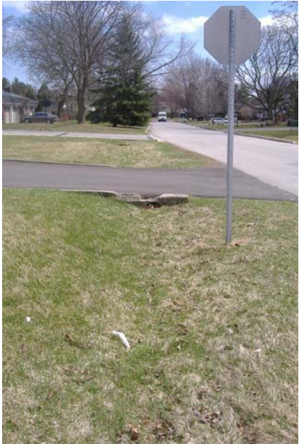
Photo 28: Looking south on Tracina at Hixon. Note filled ditch/culvert.
