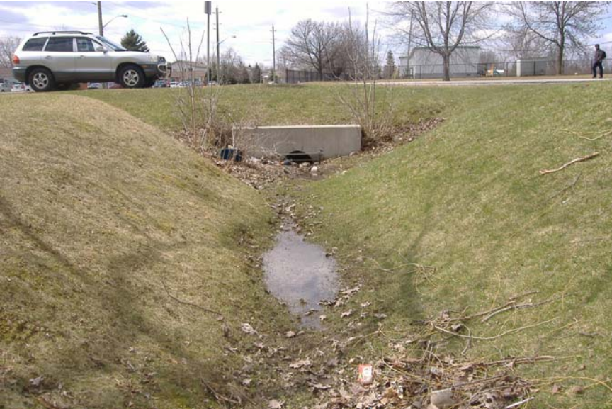
Photo 44: Looking upstream at culvert outfall. Note sedimentation and ponding.
