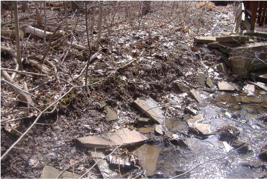
Photo 53: Looking at bank erosion adjacent to end of concrete lined channel behind Hixon Street.
