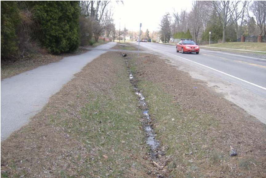
Photo 83: Looking east along north ditch of Lakeshore Road. Note standing water and erosion/rutting.
