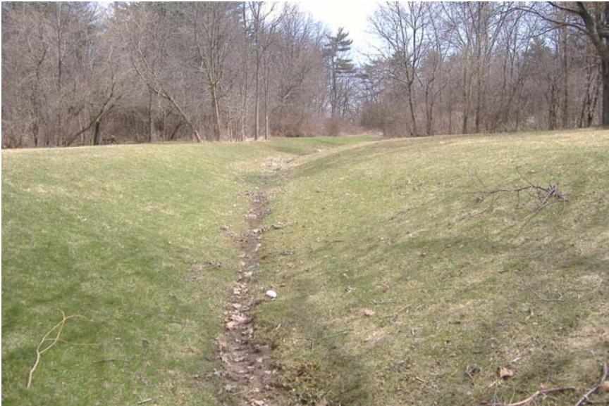
Photo 45: Looking downstream at outfall ditch. Note reverse slope.
