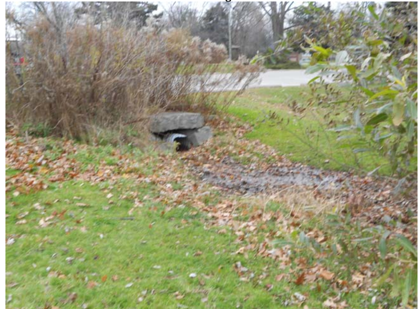
Photo 4: Looking upstream at culvert crossing of parking lot. Note standing water.
