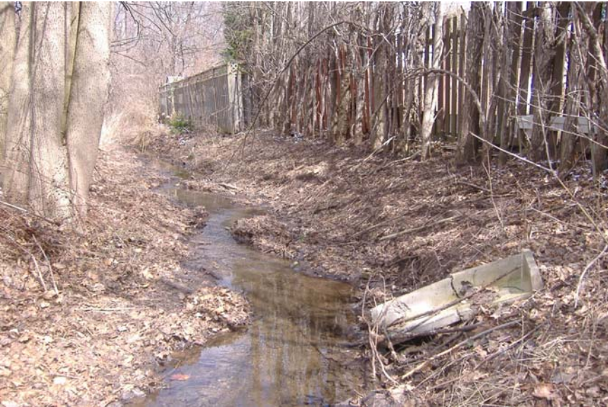
Photo 34: Looking downstream from Woodhaven Park Drive. Note minor bank erosion.
