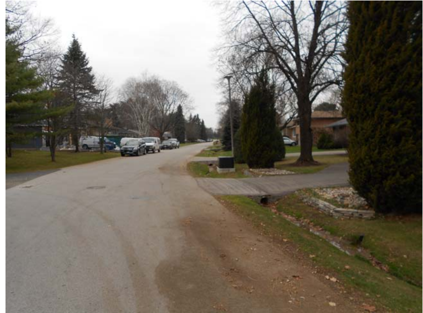
Photo 14: Looking upstream along east ditch of Westminster Drive.
