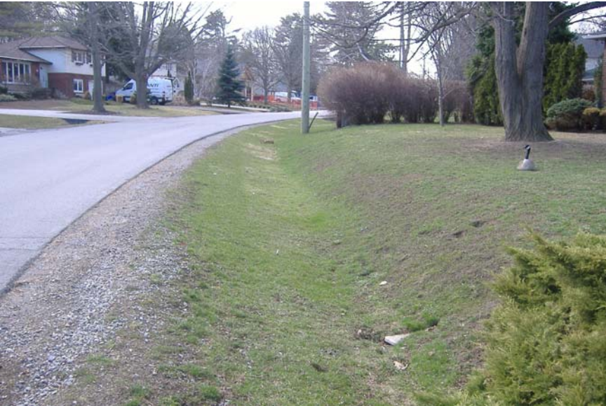
Photo 82: Looking along east ditch on Sandwell Drive.
