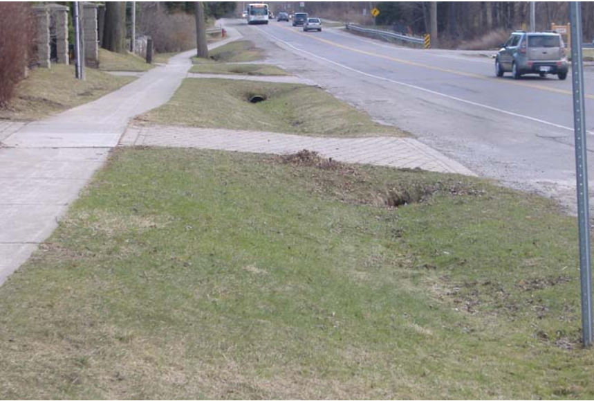
Photo 88: Looking west along south side of Lakeshore Road. Note beginning section of ditch and obstructed culverts.
