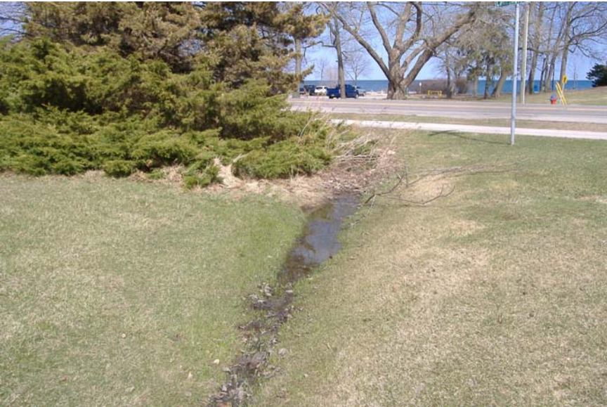
Photo 66: Looking downstream towards Lakeshore Rd from Woodhaven Park Drive. Note standing water & channel obstruction from vegetation.
