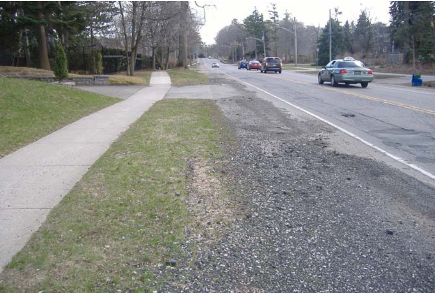
Photo 86: Looking west along south side of Lakeshore Road. Note lack of ditch and damage to roadway.
