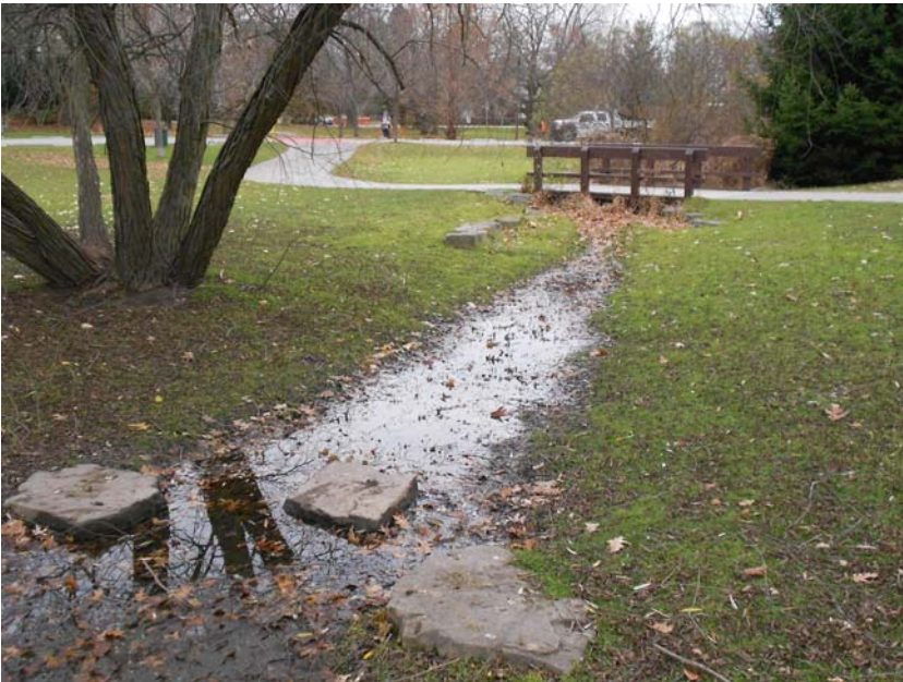
Photo 3: Looking upstream at channel and pedestrian bridge. Note standing water.
