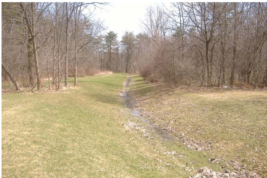
Photo 46: Looking downstream at outfall ditch. Note flat grade and standing water.
