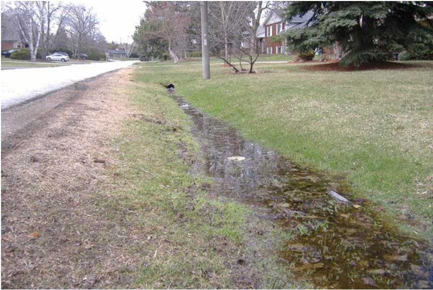
Photo 29: Looking north on Tracina at Hixon. Note standing water in ditch.
