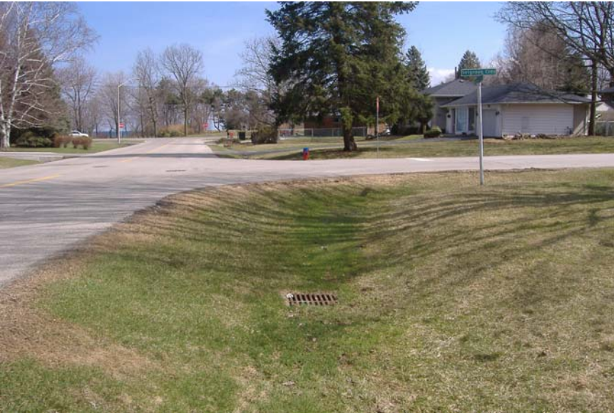
Photo 58: Looking south along west ditch of Woodhaven Park Drive at Selgrove Crescent. Note wet grass.
