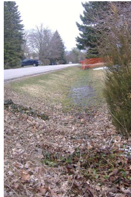
Photo 33: Looking south-east along west side of Willowdown Road. Note debris blockage of catchbasin & standing water further upstream.
