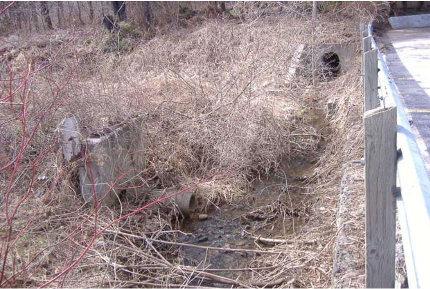
Photo 76: Looking upstream at municipal storm sewer outfall and unknown smaller outfall from WWTP site.
